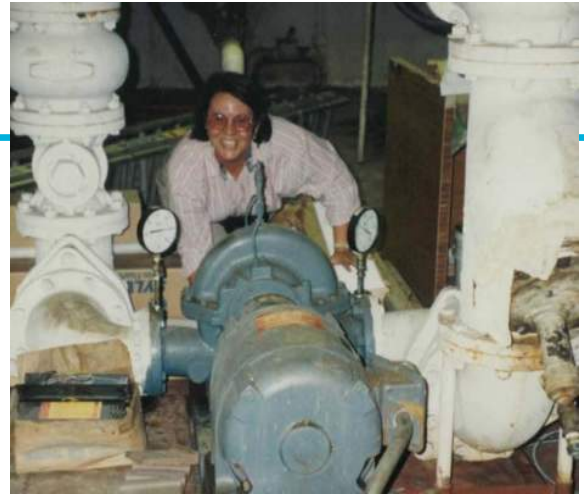
Terri in a mechanical room, 1994
