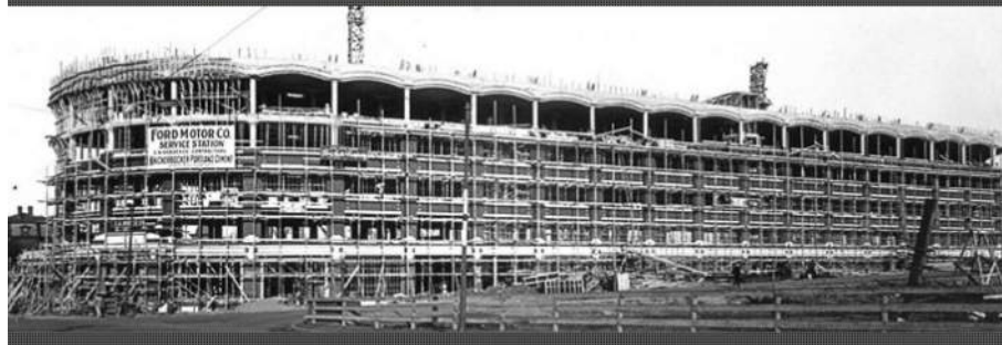
Top Left: Ford's Cambridge Assembly's central hall; parts arrived by rail from Ford's plant at Highland Park, Michigan. In early years, branch assembly plants like Cambridge averaged just 10 cars per day. Top Middle: Assembly-line workers mate an engine and chassis together at Ford's Model T plant at Highland Park in 1913, the year before the Cambridge Assembly opened. Top Right: Polaroid was a later occupant of the five-story Ford building and used it for manufacturing. Bottom: The Cambridge Assembly plant under construction in 1913. Beginning in 1910, Henry Ford built Model T plants throughout the country; assembling cars near regional markets greatly reduced shipping costs. All photos courtesy of Ford Motor Company Archives and the Cambridge Historical Commission
