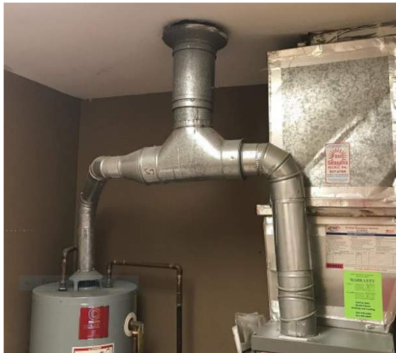
I won't tell you this pizza shop is still in business. Not saying where. It does work right? Doesn't the smaller one belong tied in above the bigger one? Nope. Equal heights with this sort of bullhead tee work fine.
