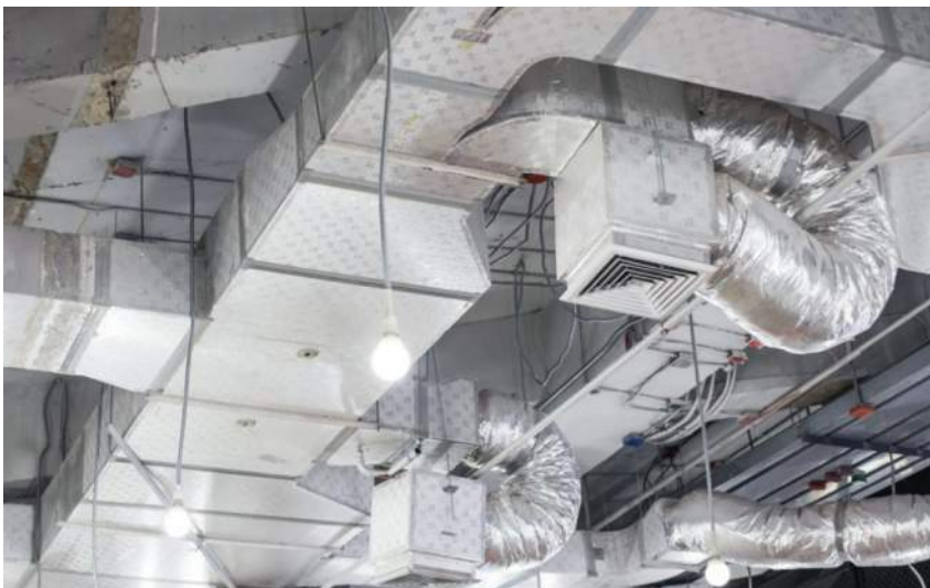
My all-time fav is flex duct on exposed applications. I would point out this is at a place of higher education. Left me wondering. At least they color coordinated the silver.
